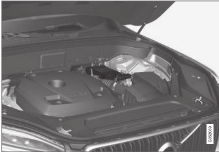
The support battery is located in a box next to the strut tower.
